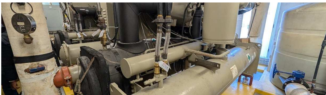
A penthouse chiller plant found running both machines at 100% around the clock, at any load. The finding that reframed an entire engagement.
