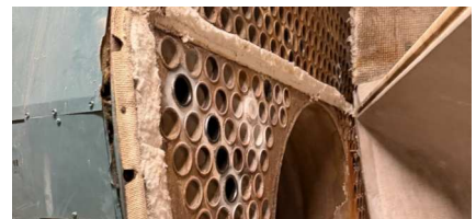
Boiler tubesheet, opened
